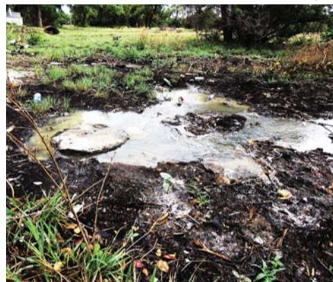
Sewage water boils from blocked system, through several manholes and flows down towards the local stream.
