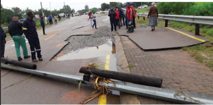
The aftermath of the devastating flash floods in Phokeng.
