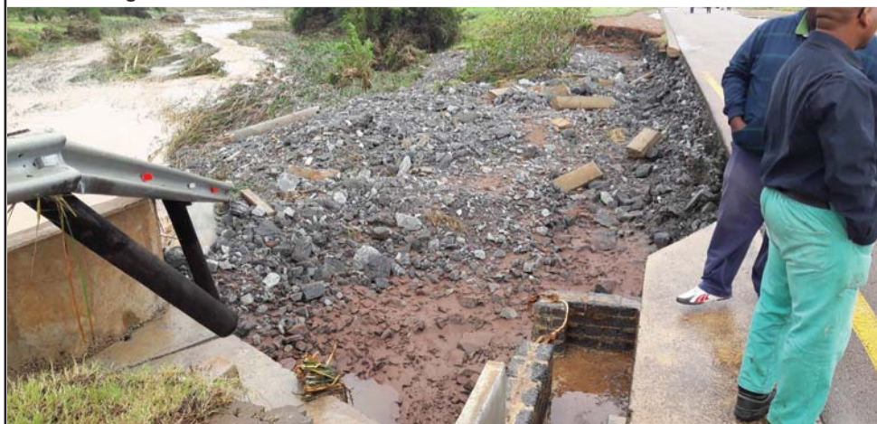
Road swept away, Phokeng, close to the Royal Bafokeng Sports Stadium.
