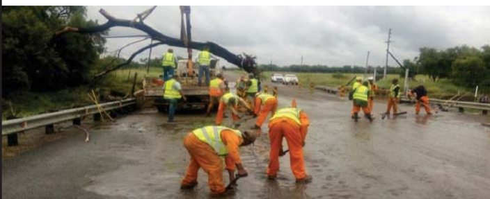
One of the many roads in the North West Province that were closed due to heavy rains. Reported on 23 February 2017: N4 between Swaruggens and Rustenburg has been re-opened.
